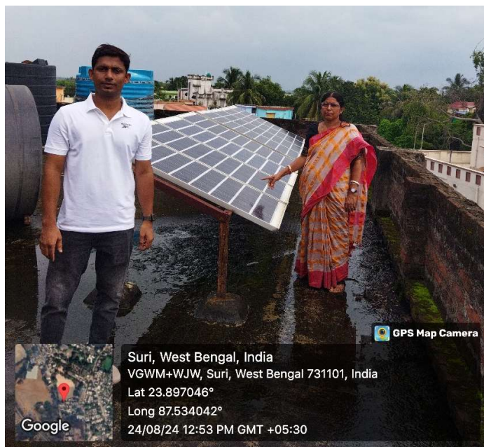
Solar panel on the rooftop of Girls' Hostel
