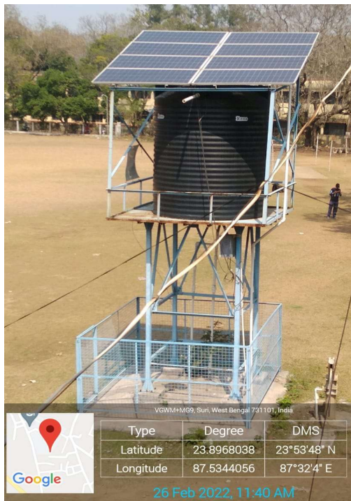
Solar-powered water pump
